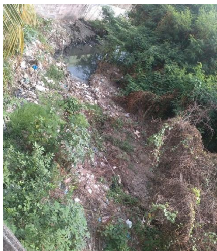
Mugalivakkam canal near sabari nagar filled with silt
