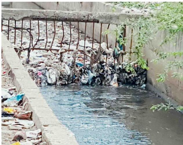
Canal flow blocked with garbage near Cowl Bazar
