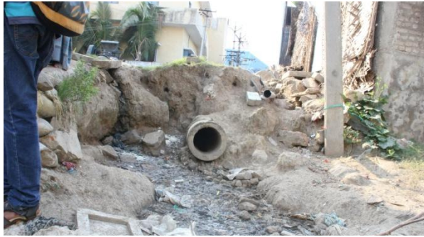
Metro water’s pipeline into canal to discharge untreated waste
